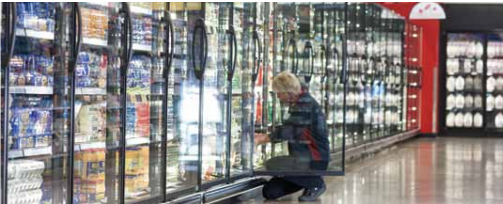
Refrigeration uses the majority of energy in food stores and represents the greatest opportunity for enhanced energy performance.
